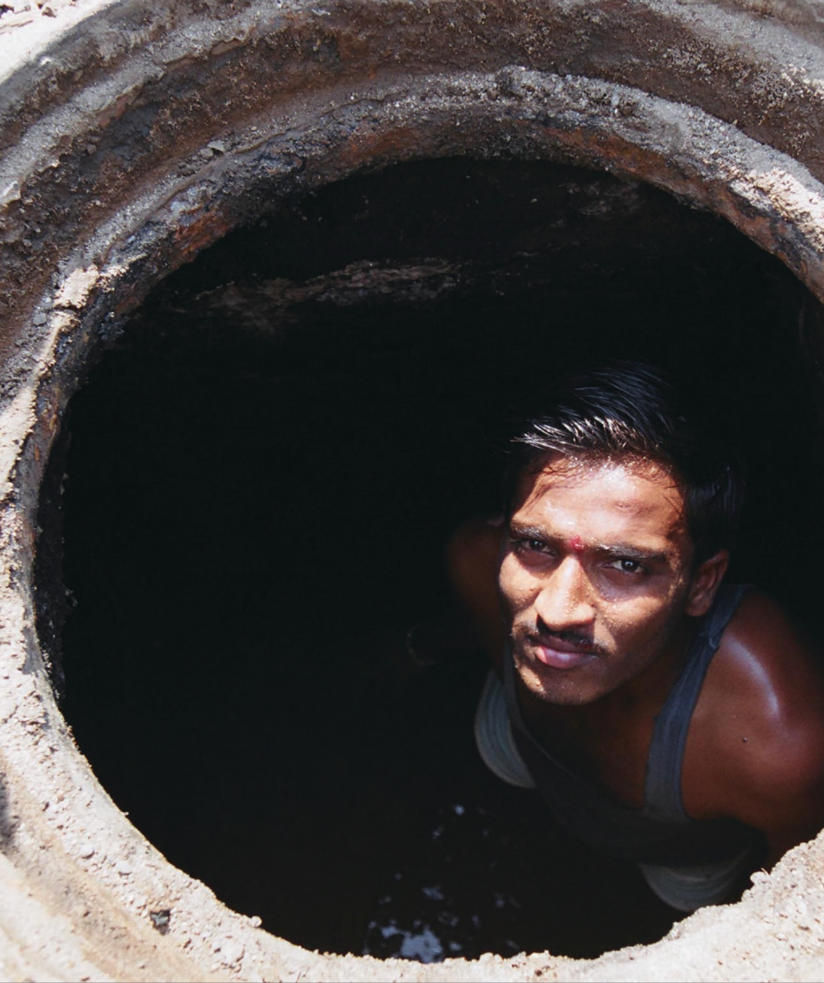
Prakash, sewage worker in Hyderabad, works in the sewer without any protection—no gloves, no suit, no boots. He uses his hands and feet to scrape and clean out the sewage pipes. India, M. Crozet, 2002. © ILO. Used with permission. Permission required for reuse.
